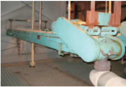
7. Sootblowers were standard on GE HRSGs burning liquid fuel
