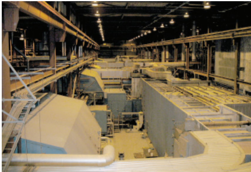
3. Gas turbines as they look leaning over the turbine-deck rail. The heat-recovery steam generator serving the first GT in the picture is to the right
