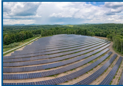
MMWEC Solar Project
